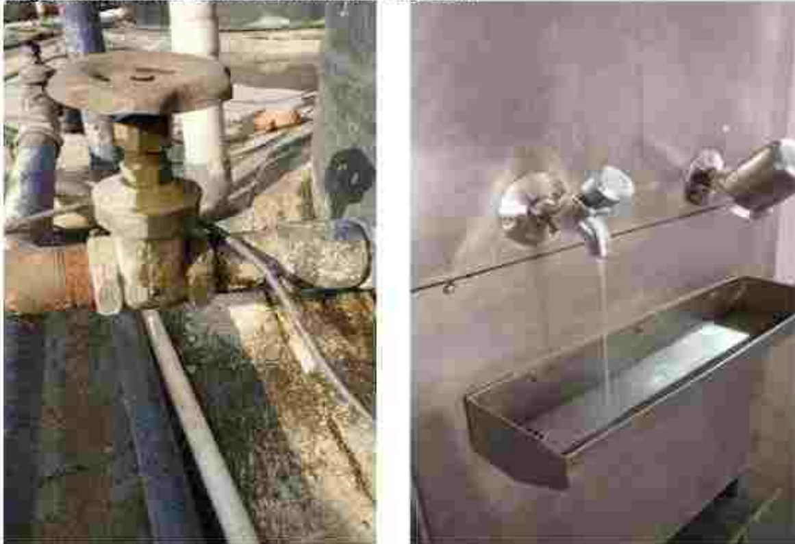
Wastage of water from the valve at roof tank & water cooler
